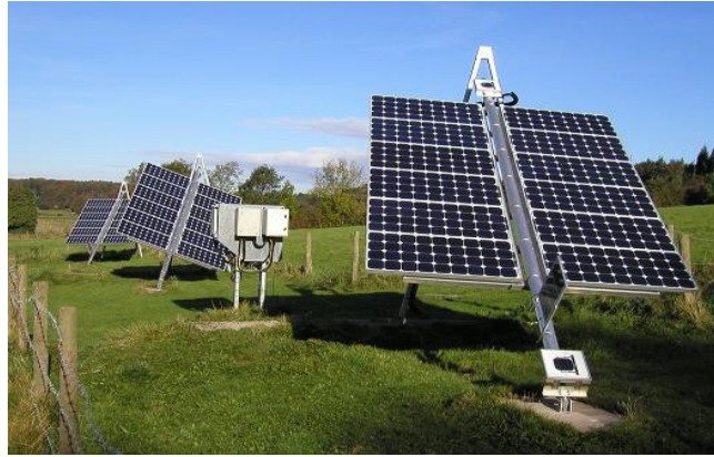
Figure 3. The interlinked, sun-tracking, 1kW photovoltaic arrays.
