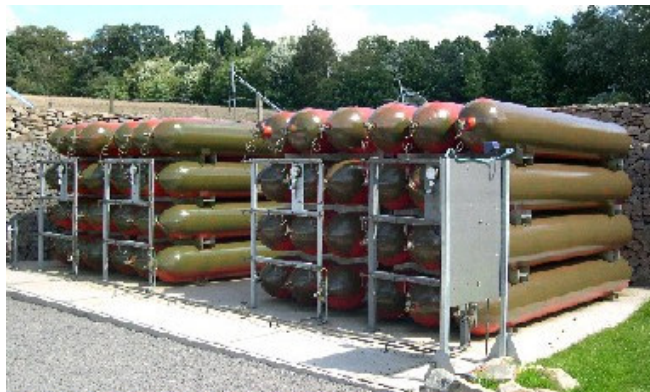
Figure 4. The bank of 48 hydrogen storage cylinders.
