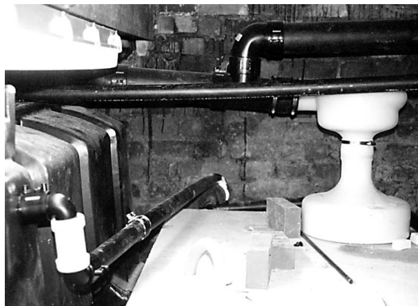
Figure 1. The bespoke composting chamber constructed from engineering brick and concrete. The white Aquatron Separator is visible on top of the chamber
