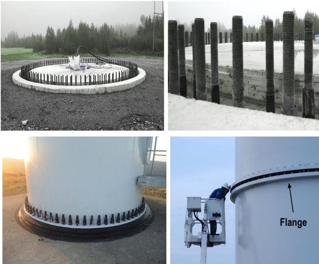
Figure 2.5 - Joint between flange, foundation and a tower section of a wind turbine [25][26]
