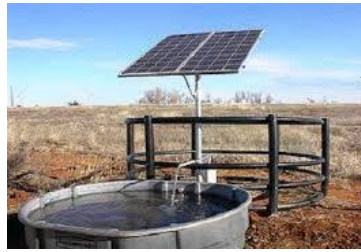
Figure 12 Application for Water pumping
